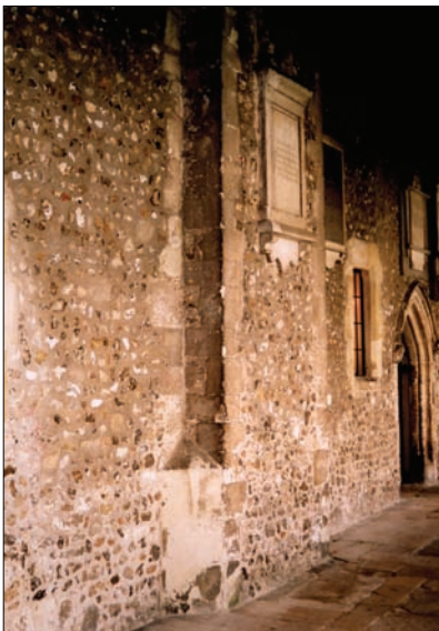
Chimneystack to the great fireplace of the Prebendaries, from the south Cloister walk
