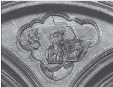
The only largely-unrestored 13th-century sculpture of the Retroquire triforium arches, one of the pair on the north
