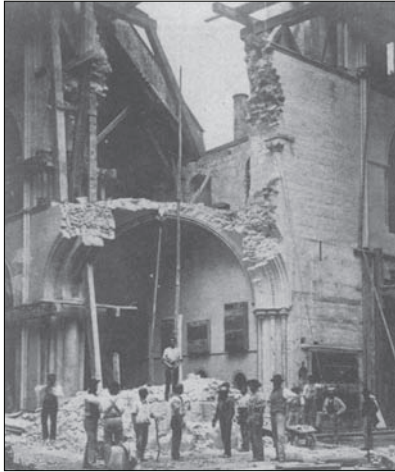
Clearing rubble from the crossing after collapse of the tower, 1861
