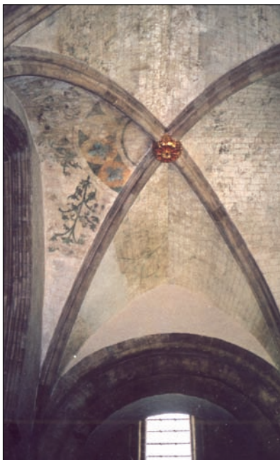
Remaining fragment of Lambert Barnard's painted vault in the South Nave Aisle
