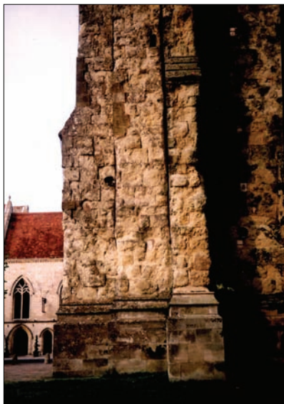
Decayed stonework on the southwest corner and buttresses of the Bell Tower
